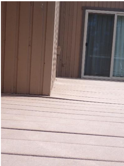
Figure 6 – Deck Warping at Exterior Wall
