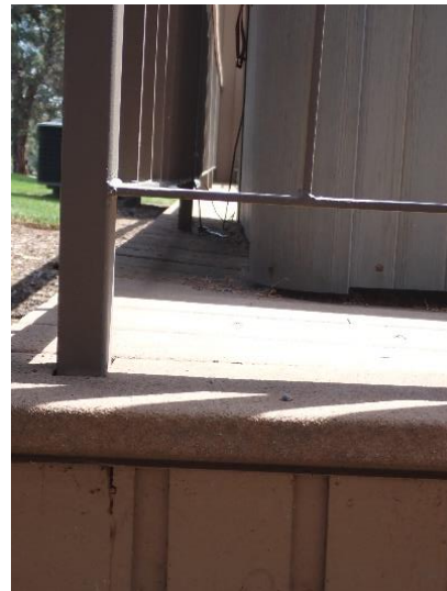
Figure 7 – Deck Warping at Hot tub
