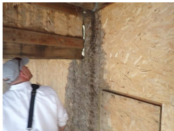
Figure 3 – Moisture Damage to Paneling and Connection
