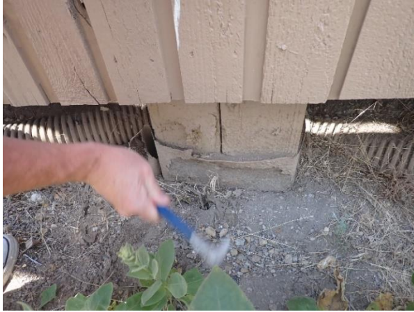
Figure 4 – Decaying Post at Base
