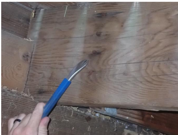
Figure 6 – Inadequate Support of New Framing
