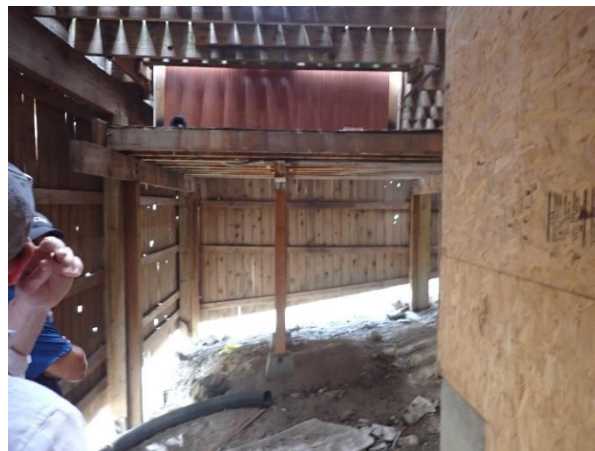
Figure 3 – No Lateral Bracing
